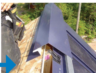
Metal roofing contractors, such as Dan Perkins of Dan Perkins Construction Inc., Ishpeming, Mich., have created and modified ridge caps to accommodate the wiring requirements of BIPV systems.
