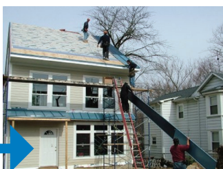
The metal roof panels are installed by a trained metal roofing contractor.
