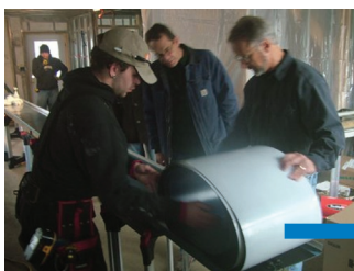
A trained metal roofing contractor installs the BIPV laminate directly onto a metal roof panel at the job site.
